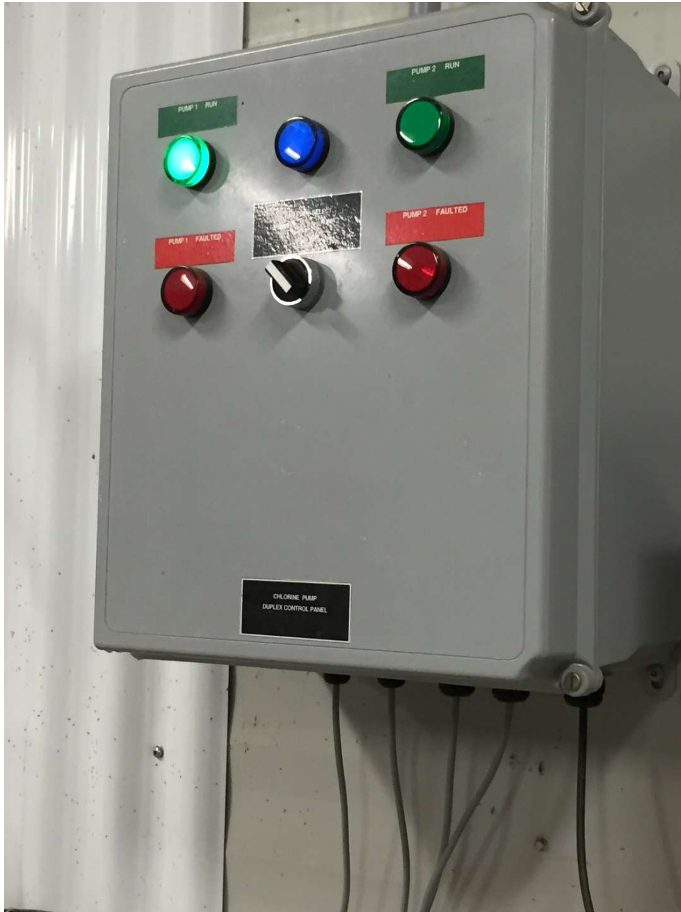
CHLORINE PUMP CONTROL PANNEL / AUTOMATIC SWITCH OVER
